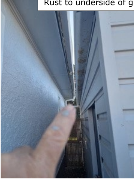
Rust to underside of gutter
