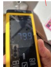
High Moisture reading
